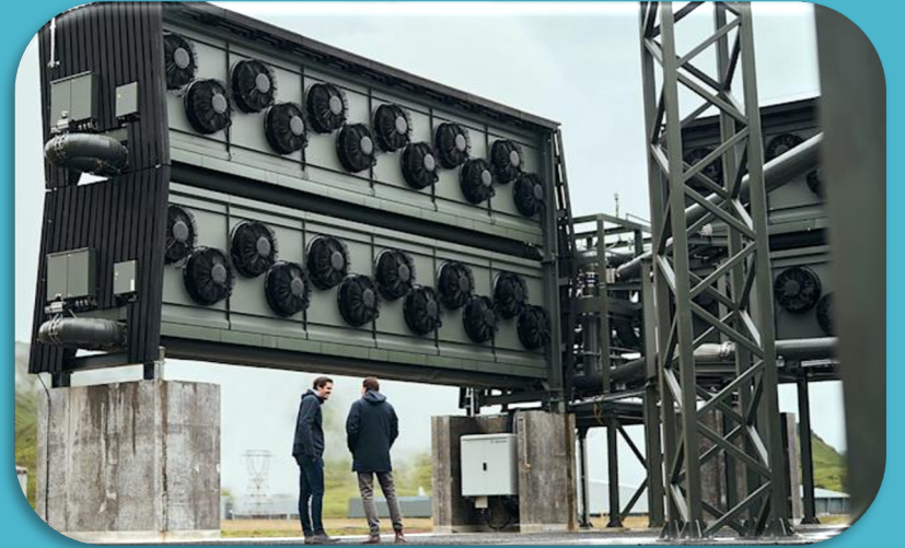
Orca, a direct air capture and storage plant
